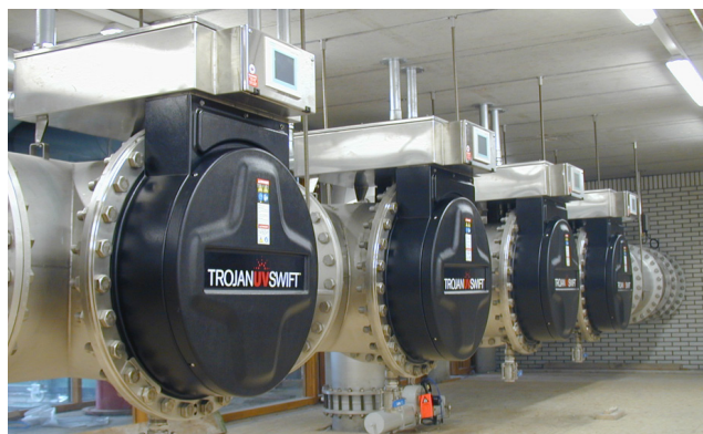
Figure 5: MP UV/H 2 O 2 installation at wtp Andijk, PWN Water Supply Company North Holland in The Netherlands
