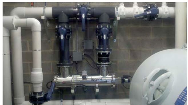
Figure 2: UV system installation in pool pump room
