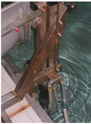
Figure 1: Corrosion of natatorium equipment due to chloramine issues.
