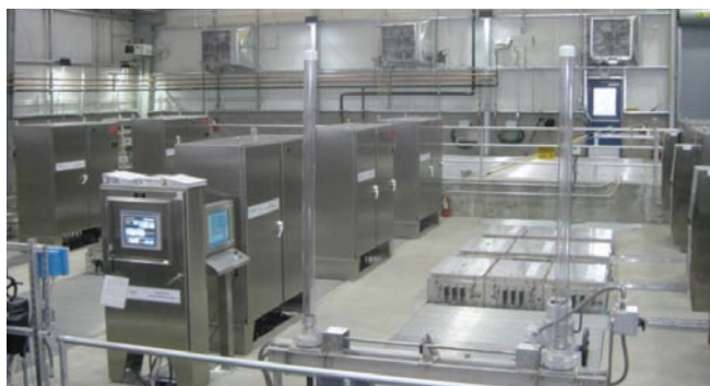
Figure 1. 135 mgd UV Disinfection Facility
