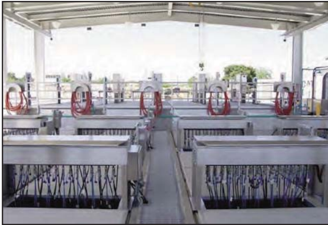
Figure 2: The plant's five effluent channels are treated with a Trojan UV3000Plus™ disinfection system. Each channel has four banks of low-pressure, high intensity amalgam lamps.
