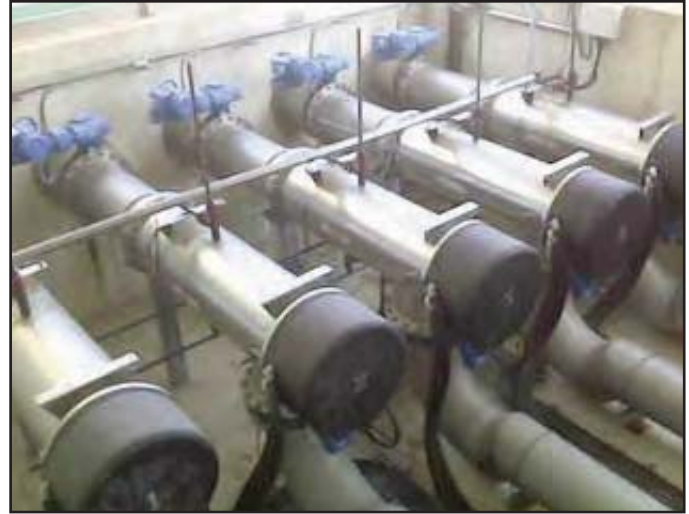
Figure 1: Five 32AL50 UVFit™ closed vessel reactors installed in parallel in Spain for disinfection of filtered secondary effluent. The reuse water was used for an irrigation application.
