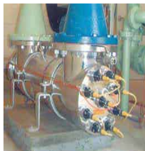
Figure 5: Wedeco – Ideal Horizons UV reactor installed at the Norfolk Spruce Road Well facility.
