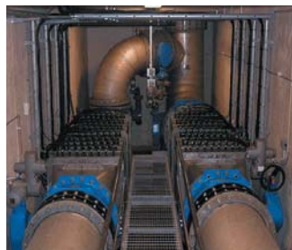
Stockholm, Sweden UV water treatment (Photo courtesy WEDECO AG Water Technology)
