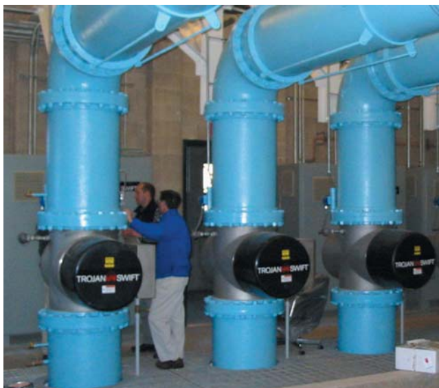
Albany, NY, USA - Medium Pressure UV System, 40 mgd (Photo courtesy Trojan Technologies, Inc.)
