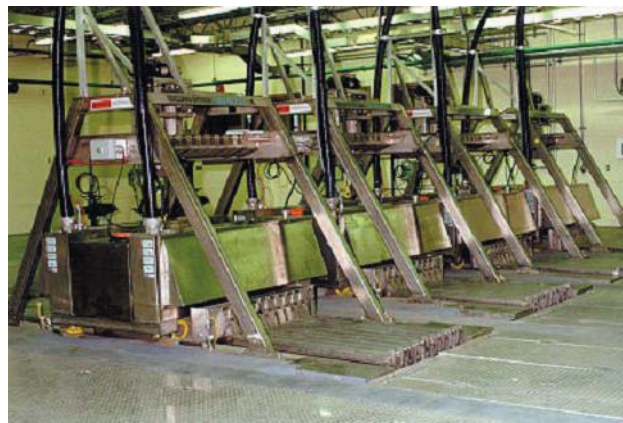
Trojan System UV4000™; 4 channels, 150 MGD flow rate
