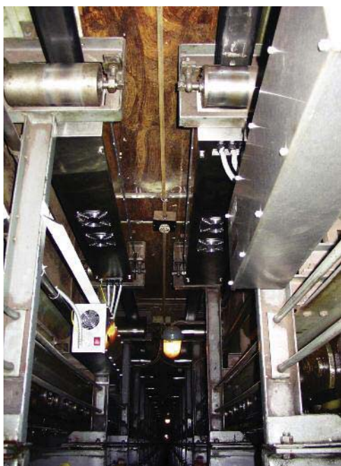
Figure 8. UV system mounted on a handrail return stretch at the "Kitai-Gorod" metro station.
